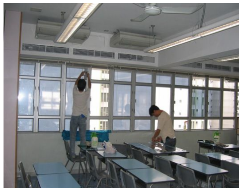
Solar Window Film in classrooms
